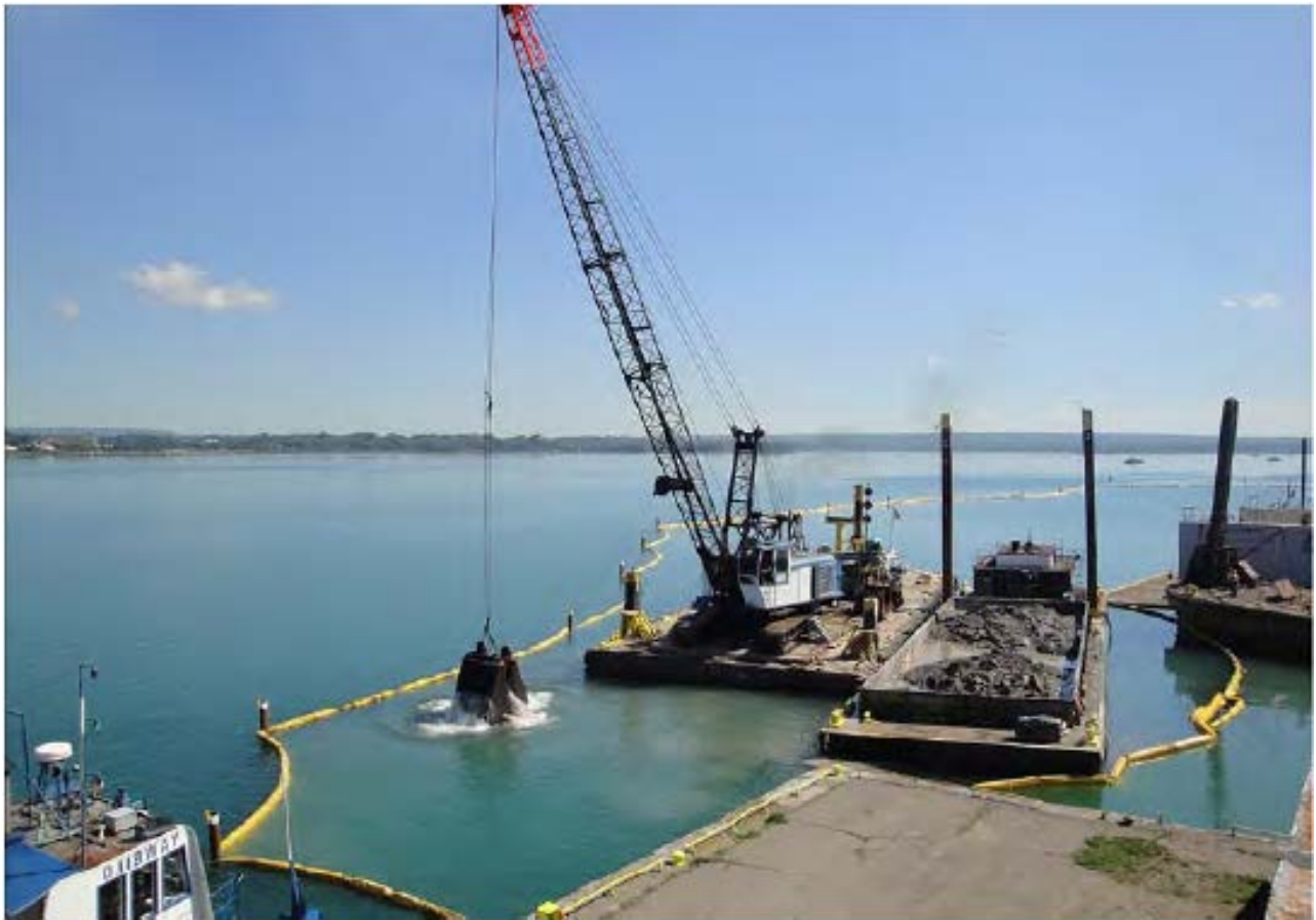
Dredging with machinery like this clamshell bucket will remove approximately 160,000 cubic yards of contaminated sediment from the portion of the Sheboygan River running from Kiwanis Park to the 8 th Street bridge as part of the Great Lakes Legacy Act dredging project. Similar equipment will remove approximately 170,000 cubic yards of additional sediment downstream of the 8 th Street Bridge.
