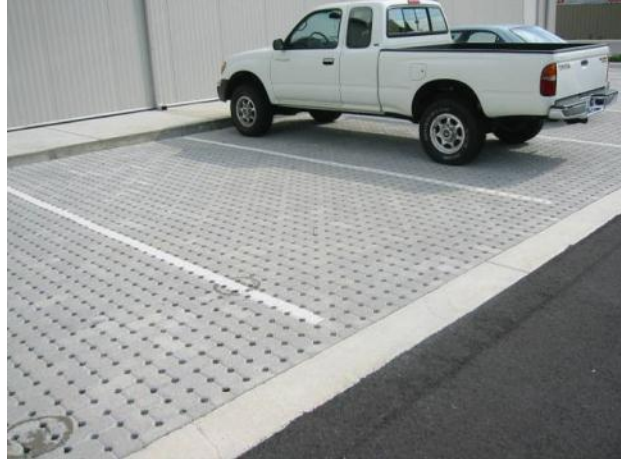
Figure 4-5. Permeable Interlocking Concrete Paver parking stalls.
