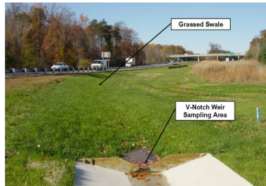
Grass Swale constructed in median on MD route 32 near Savage, MD. Courtesy of: James Stagge & Allen P. Davis, University of Maryland.
