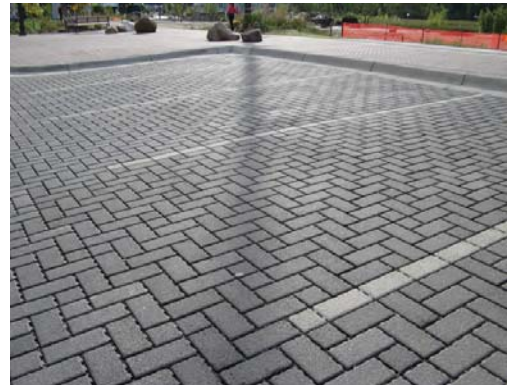
Permeable Pavers at the transit center parking lot in Mound, Minnesota. Courtesy of: Julie Westerland, MN DNR.
