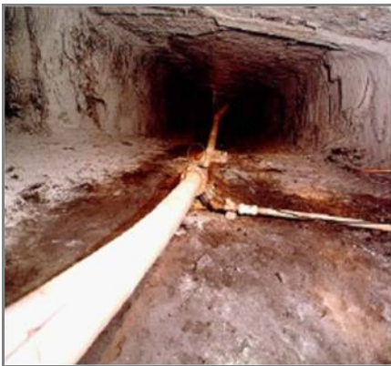
Exhibit 28: HDPE gas collection piping
