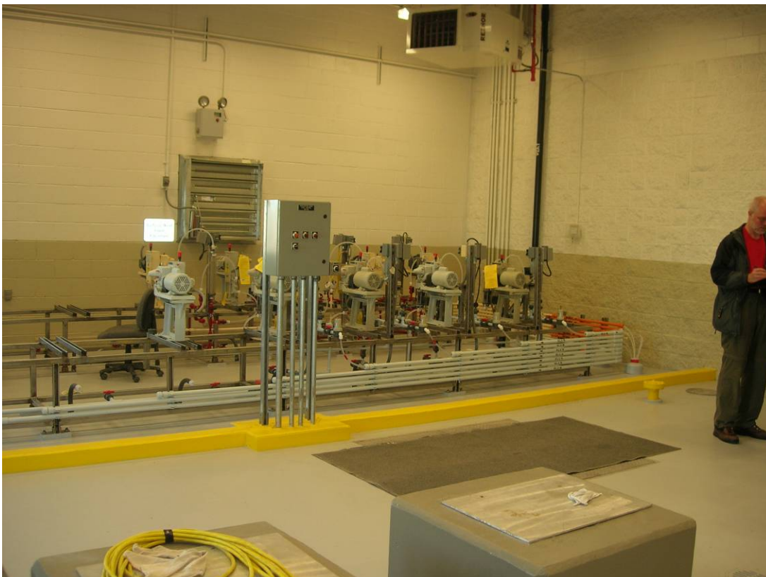
Metering equipment used for chemical addition at Pinery WWRP
