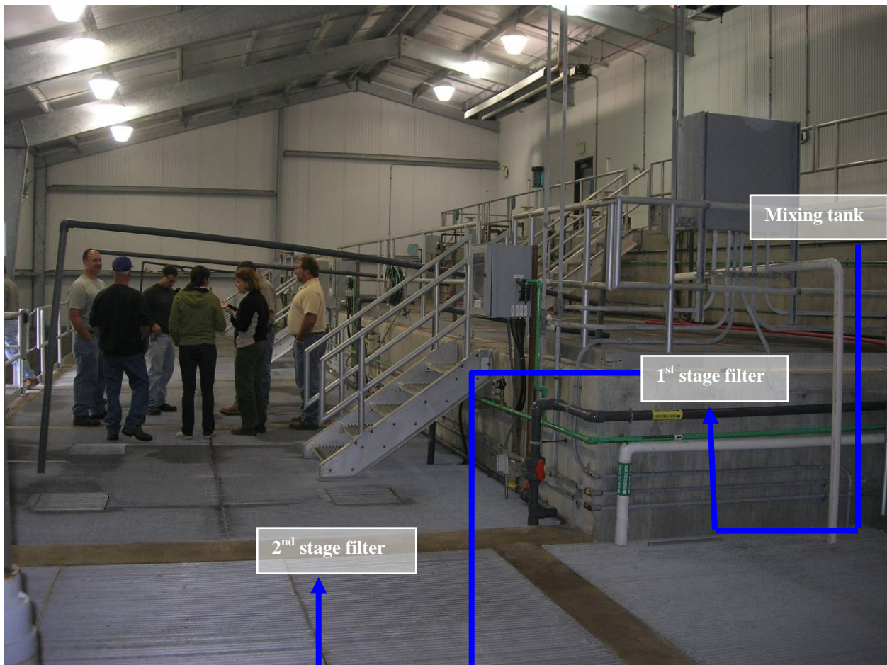
DynaSand Filters at Walton WWTP
