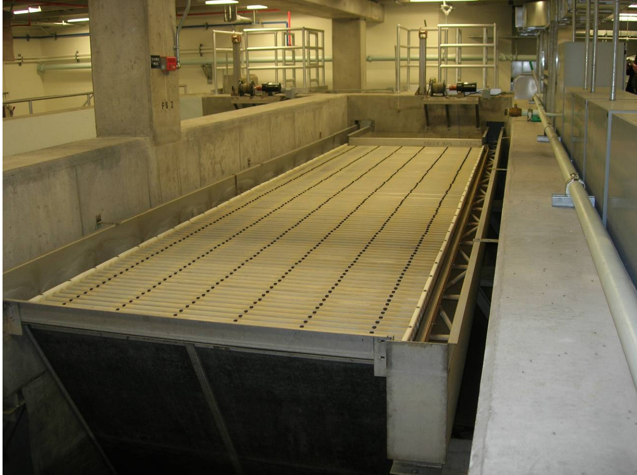
Empty rectangular clarifier with inclined plate settlers at Snake River WWTP
