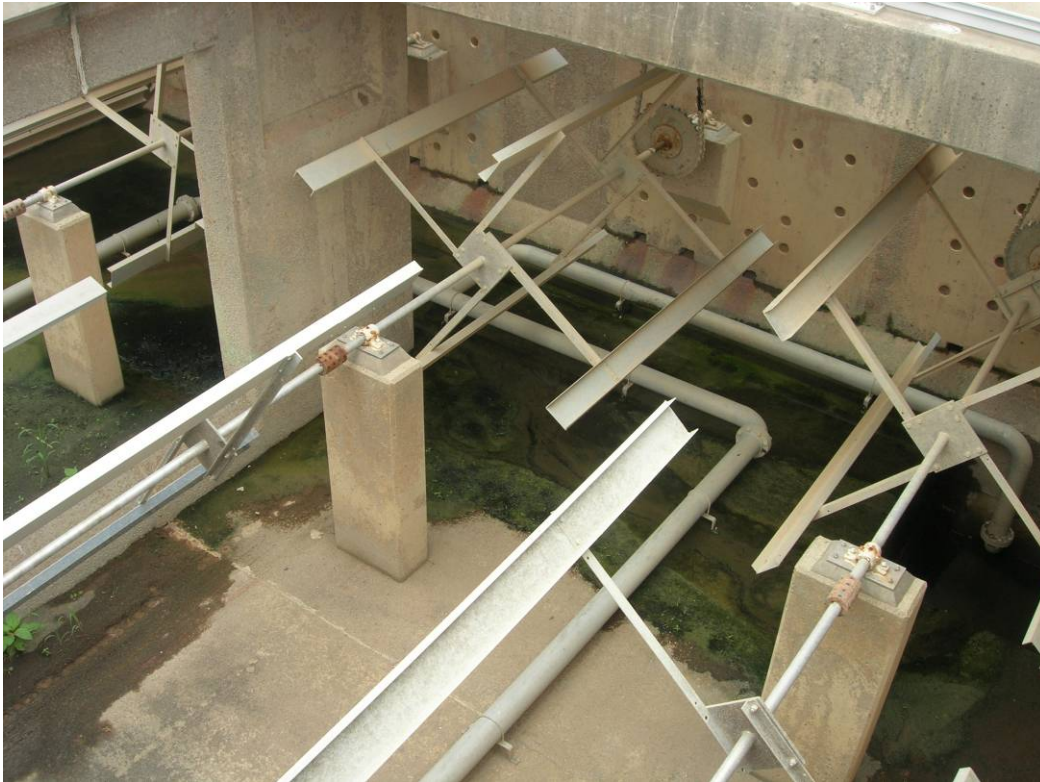
Chemical mixing paddles in front portion of sedimentation tanks at Alexandria AWWTP
