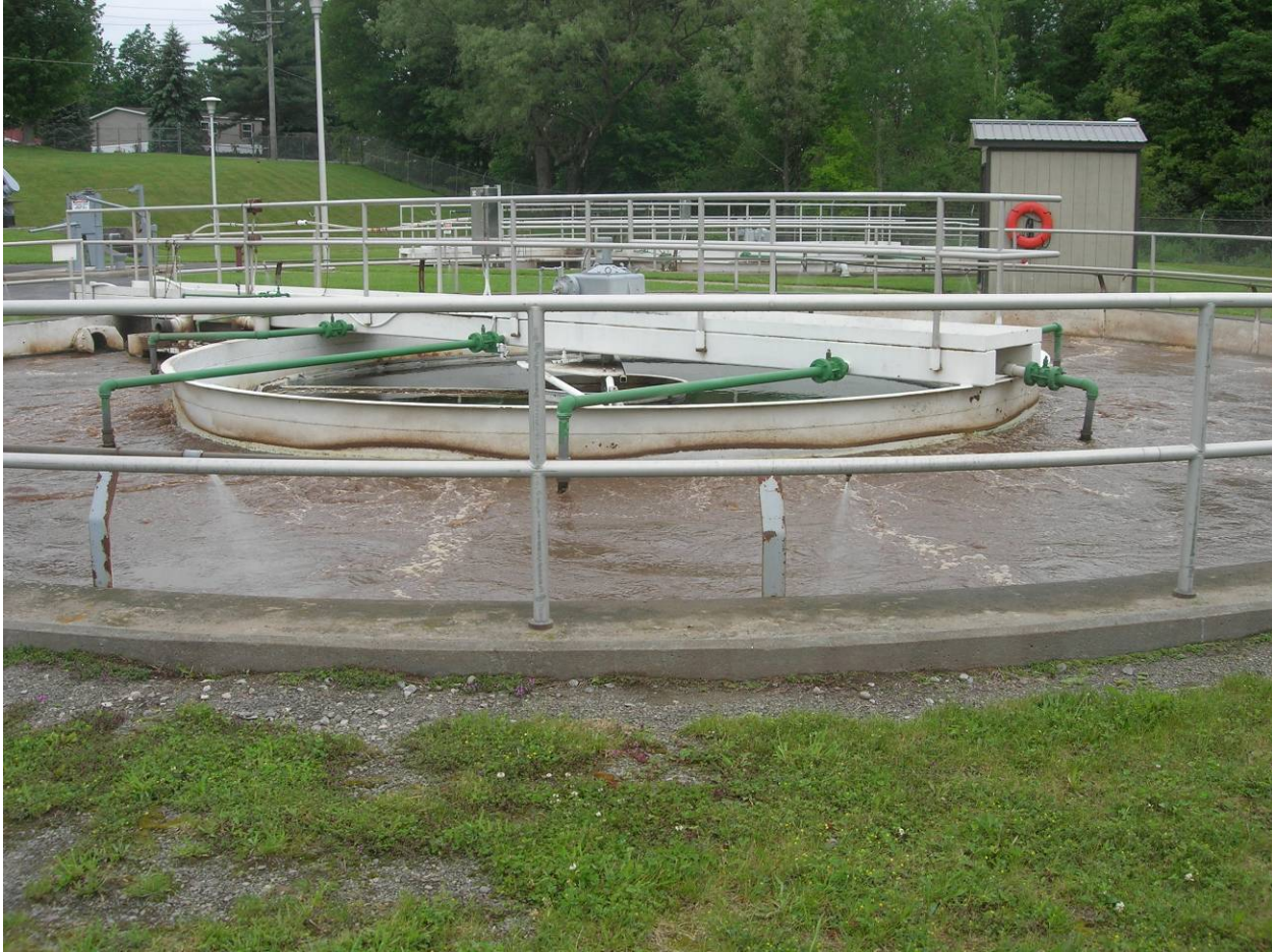
Combined aeration basin and clarifier (in center of unit) at Stamford WWTP
