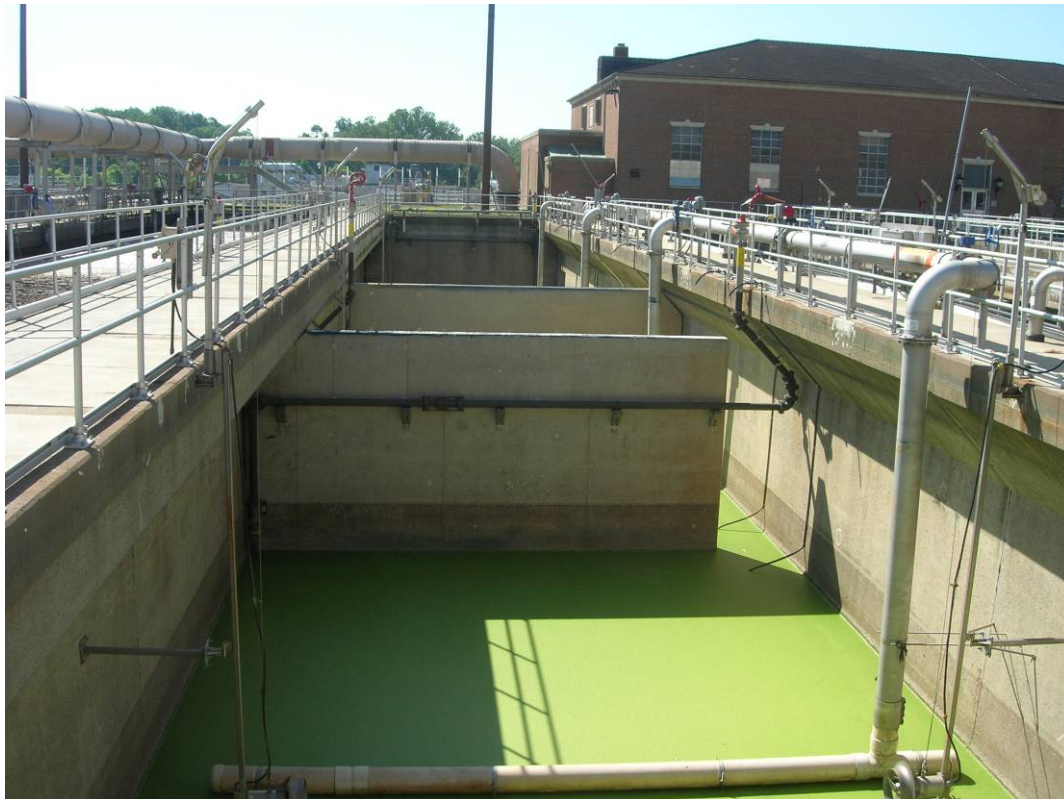
Baffles installed in wastewater contact basin (empty) to achieve anoxic and aerobic conditions for enhanced biological nutrient removal at Noman Cole PCP.
