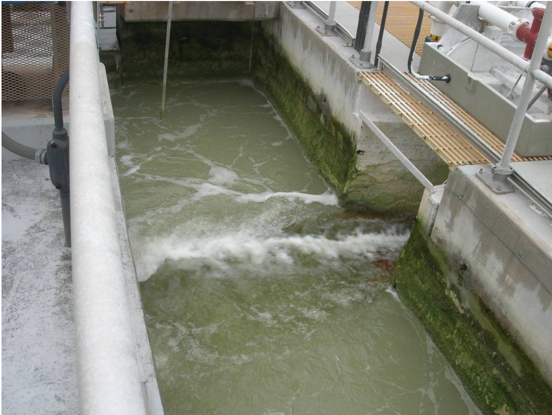
Lime slurry being mixed into wastewater at UOSA WRF
