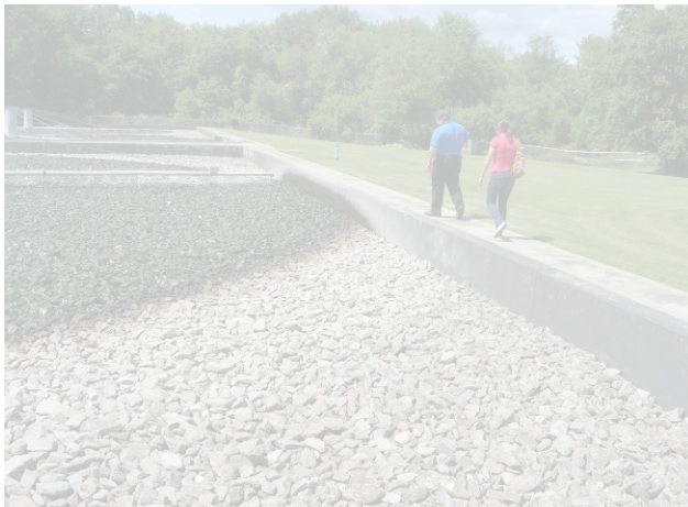
Trickling filters at Milford WWTP
