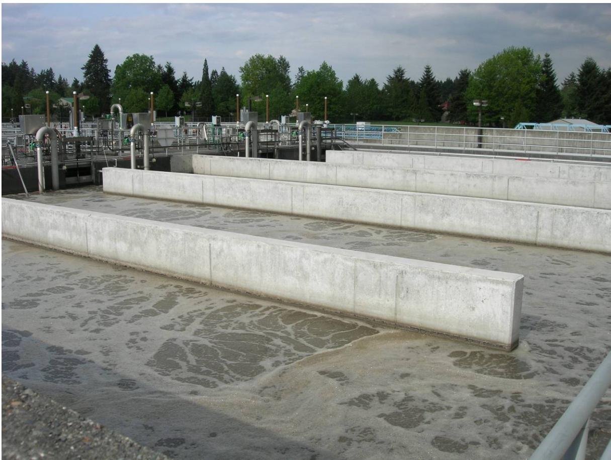
Aeration basin at Clean Water Services, Durham AWWTP. The basins at the Rock Creek WWTP may be modified in the future to also provide enhanced biological phosphorus removal.
