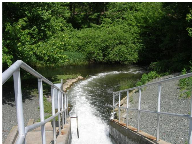
Cascading discharge structure into Charles River at Milford WWTP
