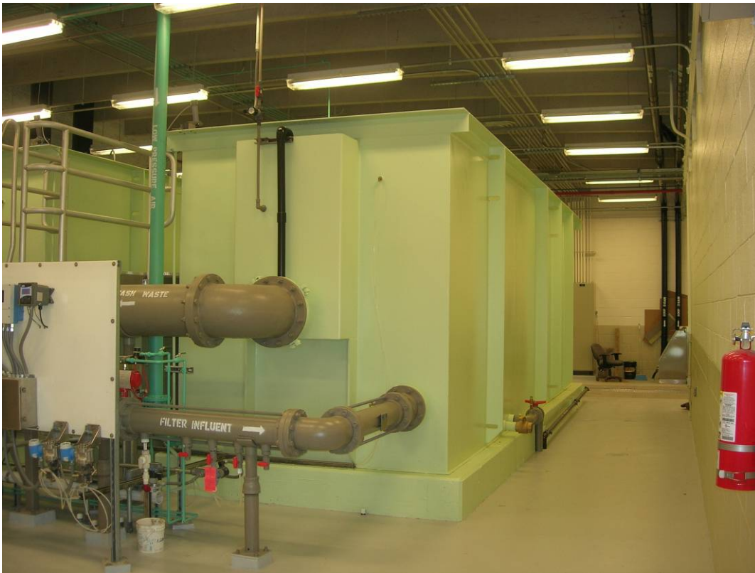
Modular Memcor Filter (US Filter Company) at Pinery WWRP. Each of these modules has a treatment capacity of approximately 0.5 mgd.
