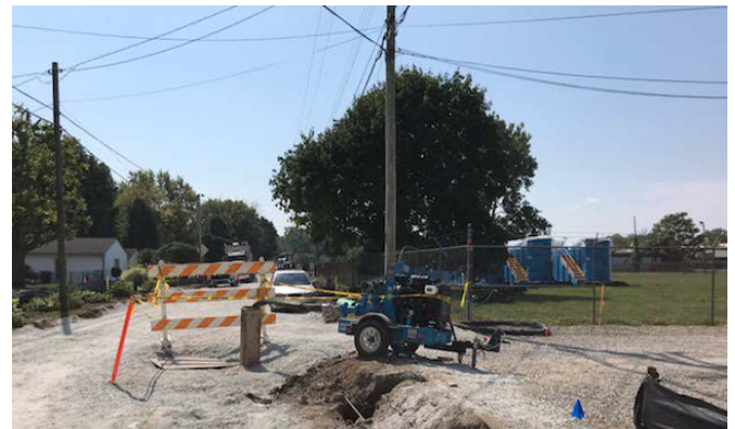
Photo #4: View looking south toward the steel dewatering well and pump & offsite blue frac tanks
