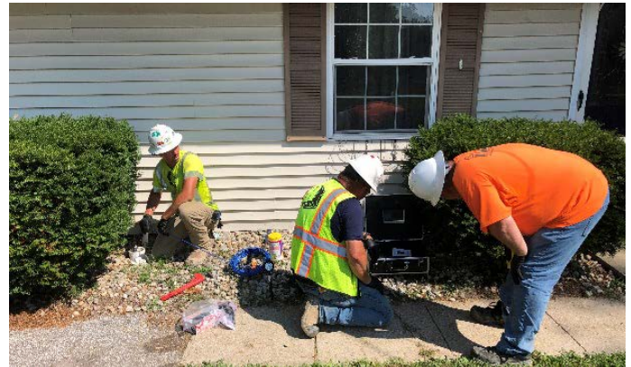
Photo #2: Sewer lateral inspection when entering from an existing exterior sewer cleanout
