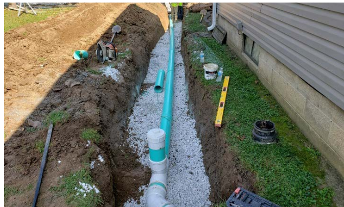
Photo #3: View looking east along a newly installed 6-inch diameter PVC sewer lateral & cleanout
