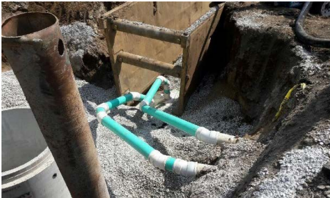
Photo #1: View of MH 250050, steel dewatering pipe, and two commercial sewer laterals
