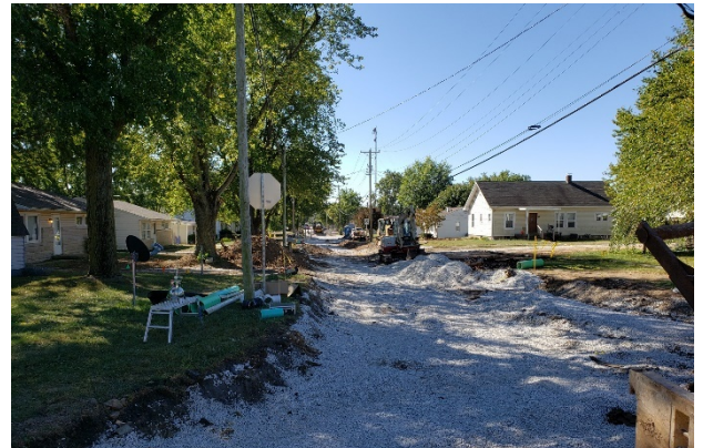
Photo #4: Looking south from Hamilton Avenue, sewer main replacement complete on Forsythe St
