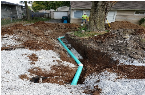
Photo #3: View looking east at new sewer lateral traversing around an existing tree
