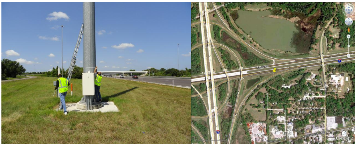
Figure E-4. Tampa EPC02 site photo (left) and Google Earth image (right).
