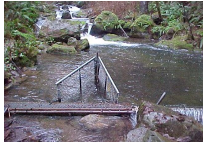
A Drinking Water Intake for a Surface Water System
