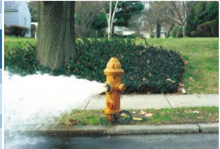
Hydrants Provide Water for Fire Suppression, Line Flushing, and Irrigation
