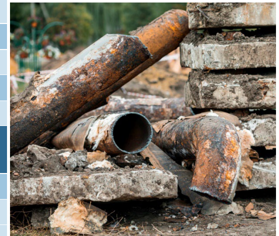
Broken old rusty pipes
