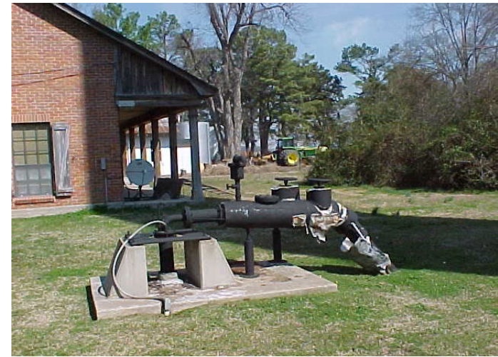
A Ground Water System Well
