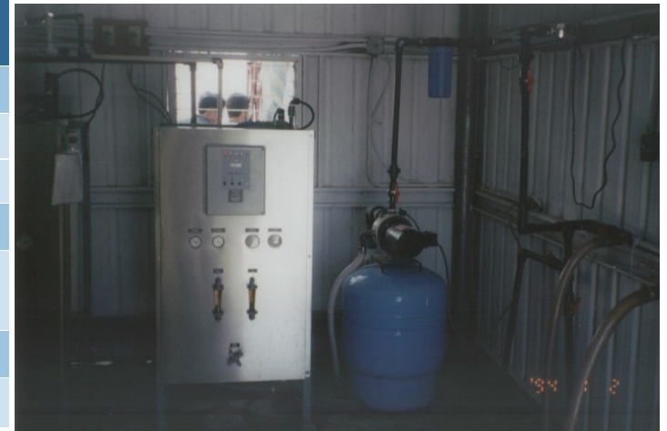
An Electric System
