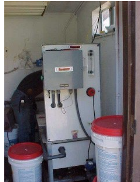
A Chlorination System
