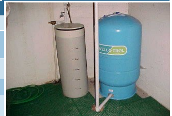
A Hydropneumatic Storage Tank
