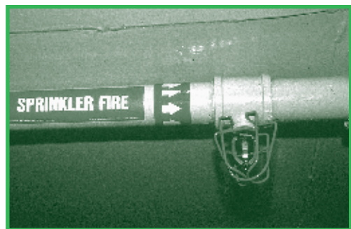
Install fire detection systems such as this sprinkler system with a sensor.
