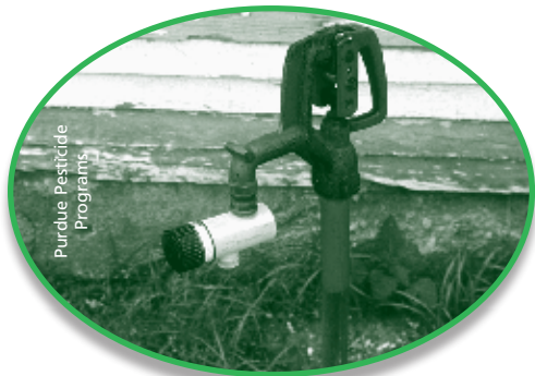
Use a backflow device when water is pumped directly from the source.
