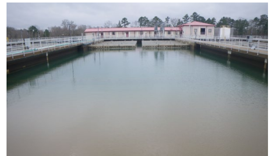
Figure 2: Sedimentation Tank at OB Curtis water treatment plant in Jackson
