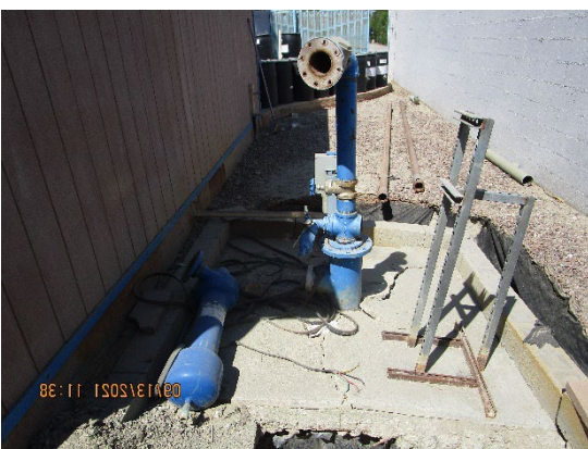
Figure 4: Remains of collapsed Well #1
