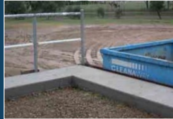
Concrete lip and container offset to prevent vehicles backing over the platform edge
