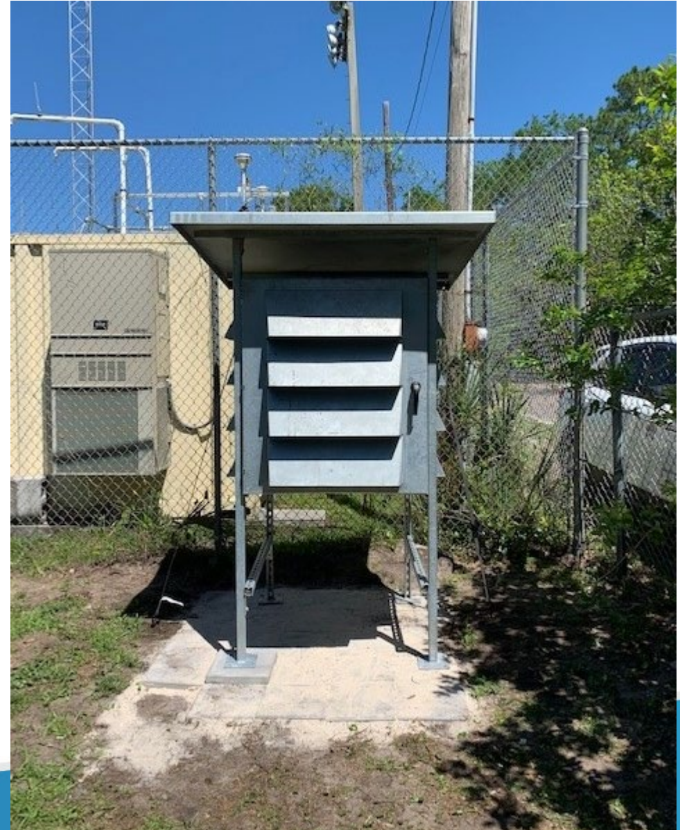
Collocation Shelter installed in Jacksonville, Florida
