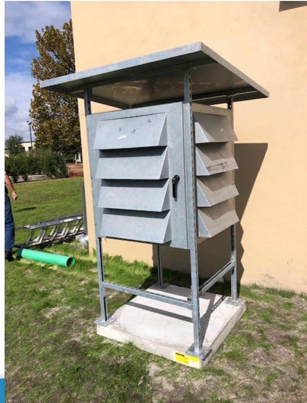
Collocation Shelter assembled in Orlando, Florida
