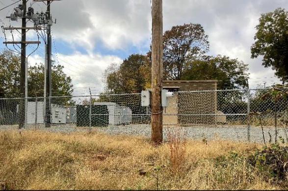
The Maple Street Substation battery storage facility providing 10 MW of power storage for the city's grid.
