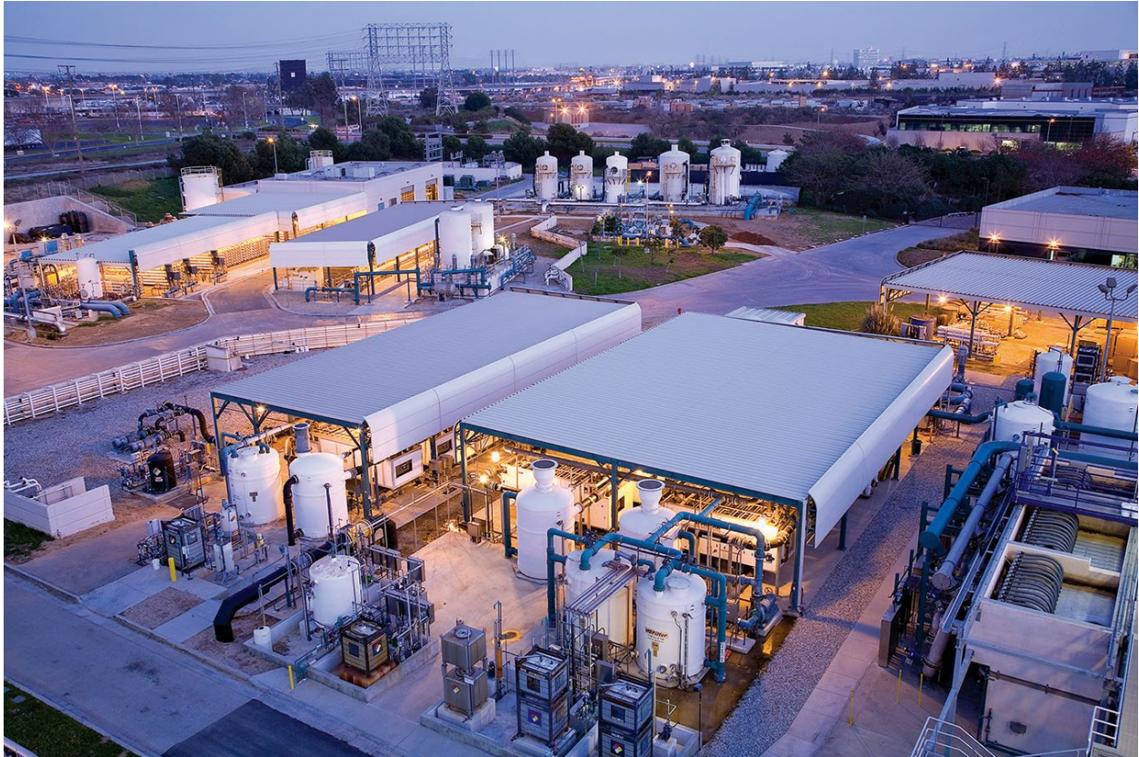
West Basin Municipal Water District's Edward C. Little Water Recycling Facility in El Segundo, California, produces five different types of recycled water for different uses including groundwater recharge.
