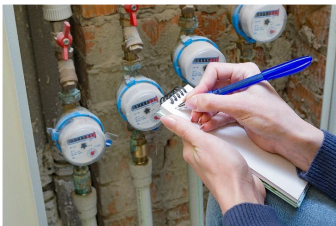
Reading facility submeters
