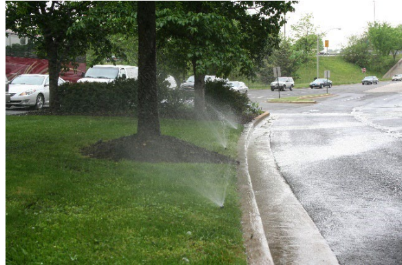
Improperly positioned irrigation sprinklers spraying onto pavement
