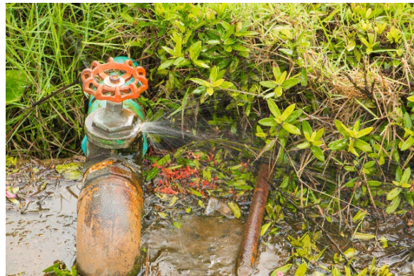
Leaking irrigation valve
