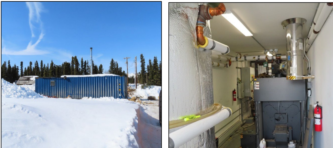
Figure 2. Mentasta's biomass heat facility, exterior and interior views. Credit: ANTHC Rural Energy.
