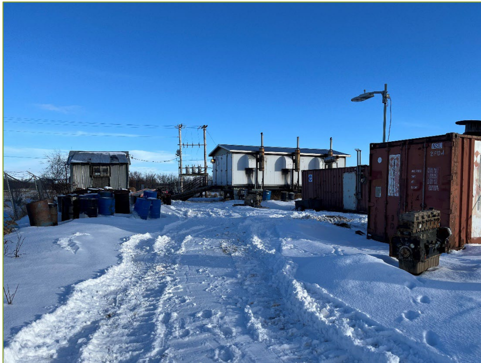
The 567 kW power plant in Napaskiak, Alaska. Credit: ANTHC Rural Energy.
