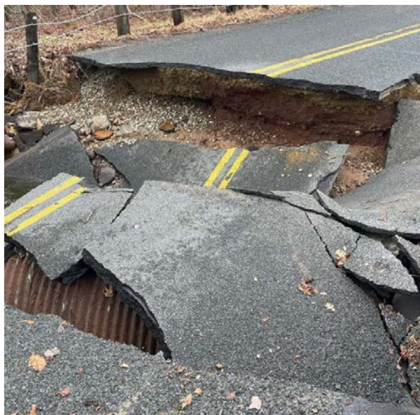
Figure 5: Storm damage in January 2024.
