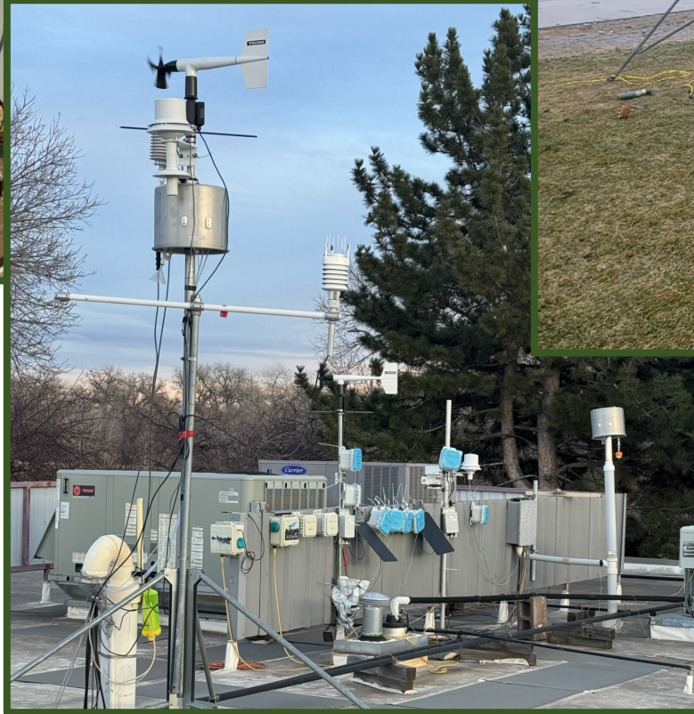
Acceptance Testing ARS Roof Fort Collins, CO
