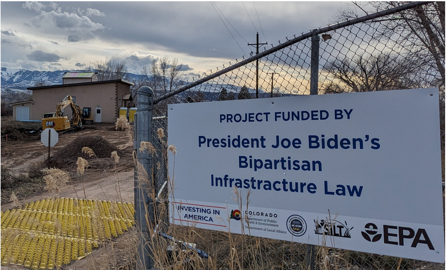
The Town of Silt, CO, received funds through the Drinking Water SRF to construct a new water treatment facility. Courtesy of EPA Staff
